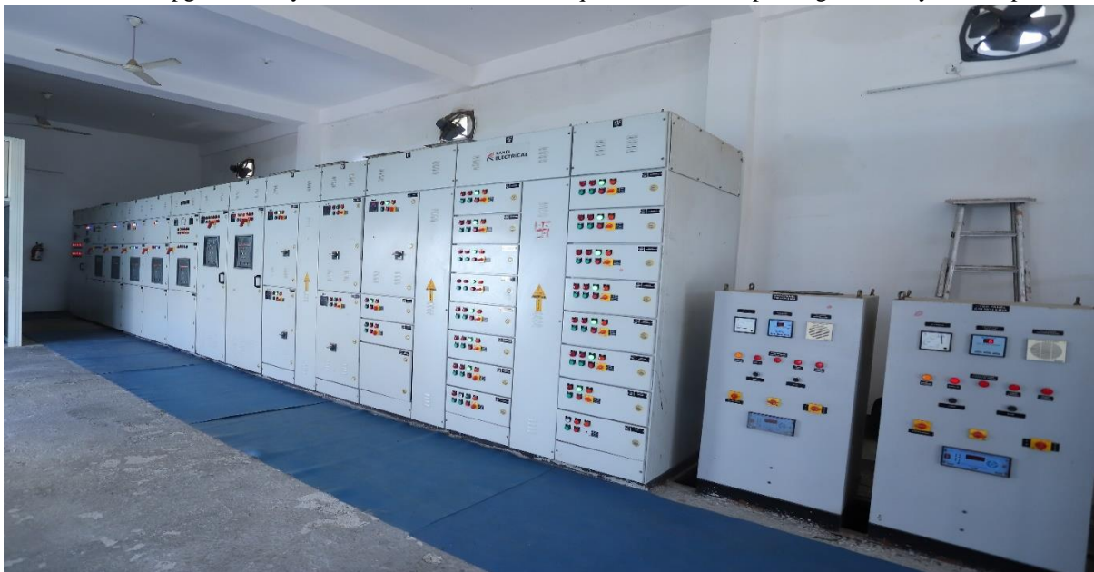
IPS Control Panels, Ghaziabad
