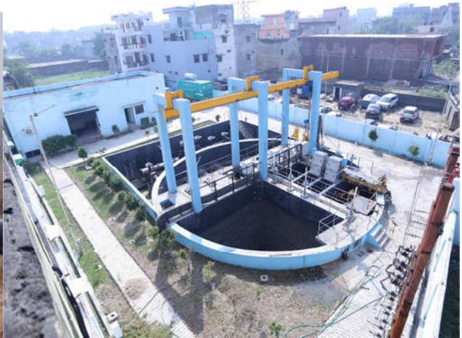
Raw Water Rising Main Unnao & Shuklaganj water Supply Scheme
