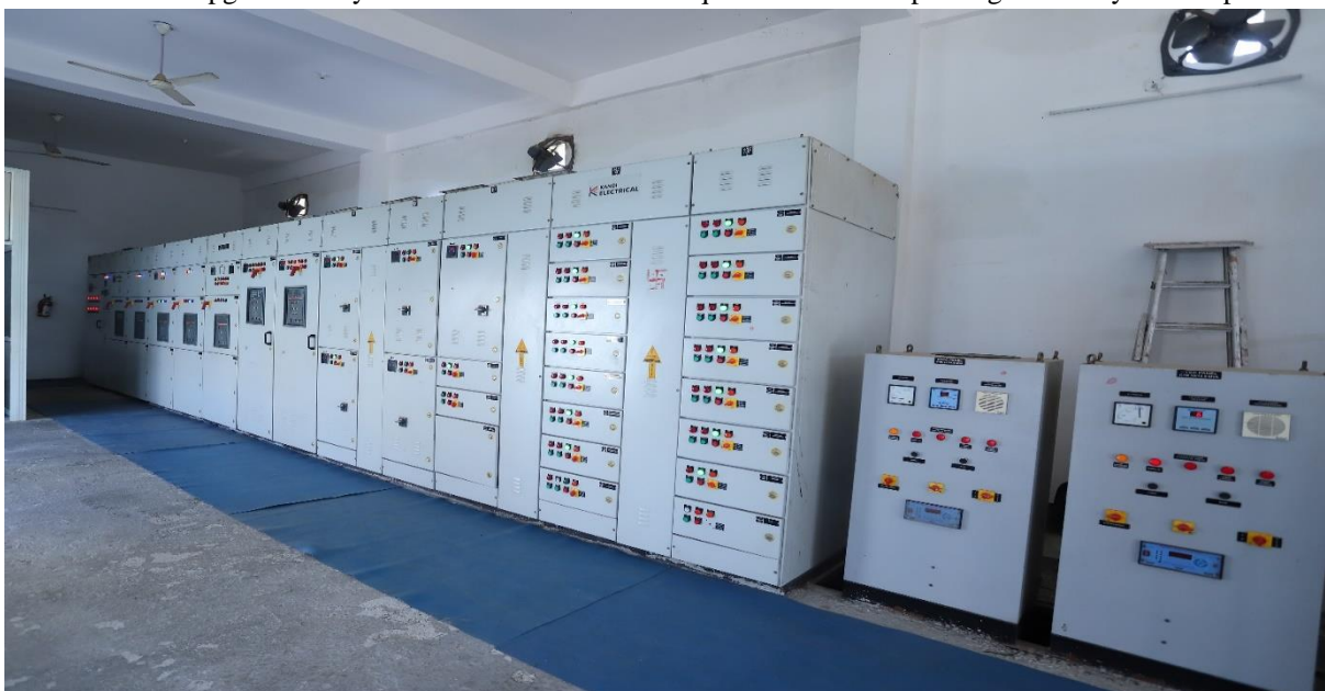
IPS Control Panels, Ghaziabad
